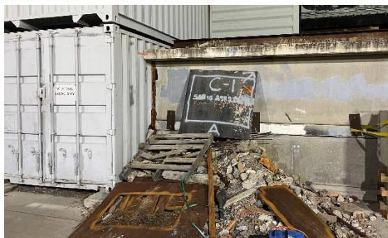
Figure 9 Pancake collapse with heavy lift for access.
